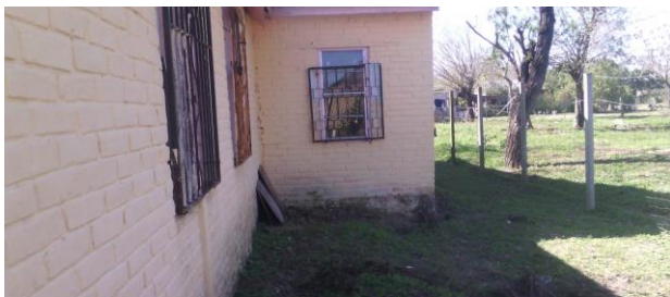
This is the wall that will be moved to the left to give more room in the sanctuary.
