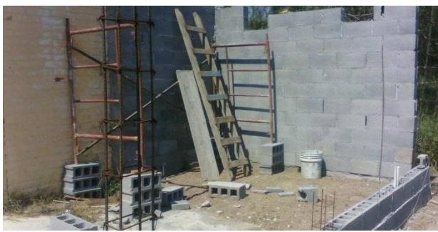
Back and side walls to the office area. The front wall will be where the cement blocks are being laid.
