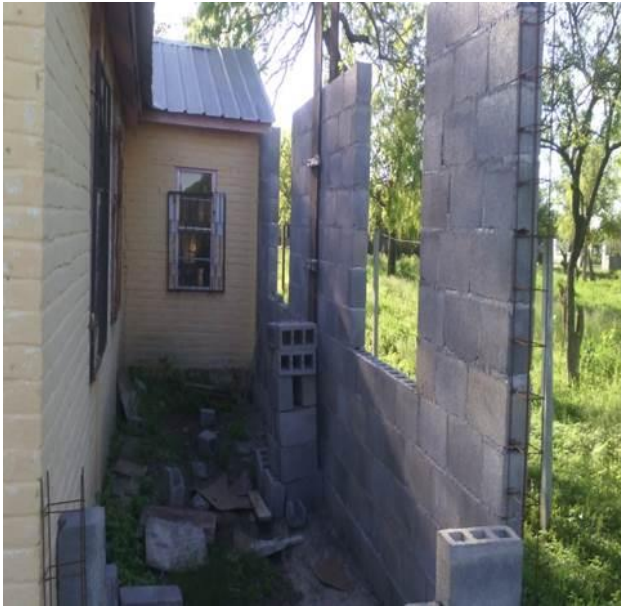
The right side of the church is being widened and an office is being added to the front portion.
