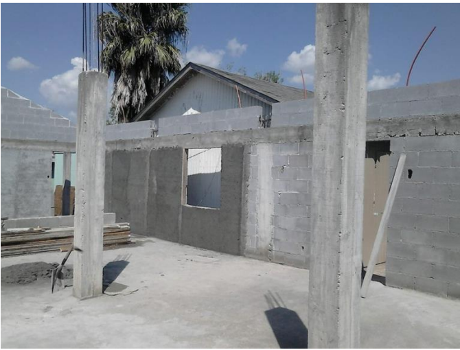
It looks like two more levels of cement block were added to the walls all around. Plaster was added to cover the cement block so they can have smooth walls inside. In this picture you can see the top of the older wooden structure off to the right.
