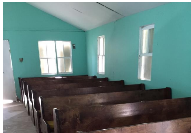
The ceiling and walls are coming apart due to the shifting of the building.
