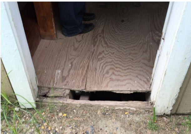
The entrance to the side door of the church. Building is shifting and there is a gap now to an open area under the building that fills up with water when it rains.
