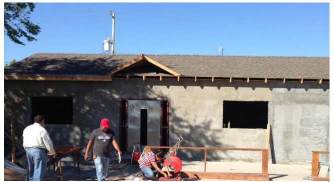
El Mesias - roof is on, walls are up, doors are being installed
